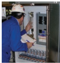
Control and Monitoring
