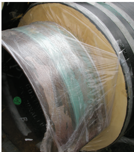
nVent provided an optimum heat management system solution through careful evaluation of the insulation systems available to the project.
